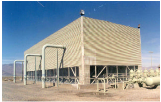
Power plant cooling tower.
