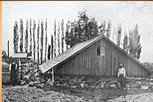
The first story of the Siard Ranch poultry house collapsed in the 1915 Earthquake. (Jones, 1915)
