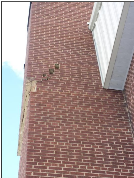
Figure 4. West wall of chimney. Note shear fracture and horizontal displacement.
