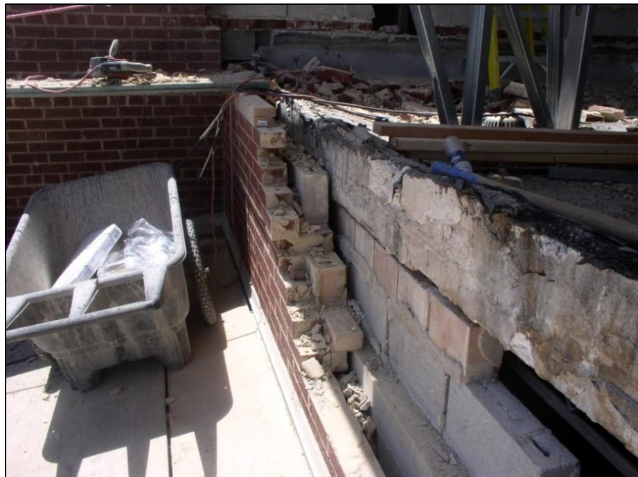
Figure 6. Delaminated brick and masonry wall at southeast corner of auditorium (roof level).
