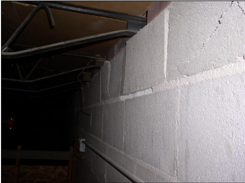
Figure 3. Common wall between gymnasium and auditorium showing fractured masonry units below auditorium roof bar joists.
